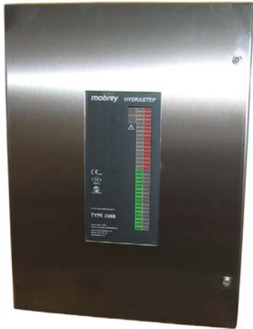
Hydrastep Control Unit
